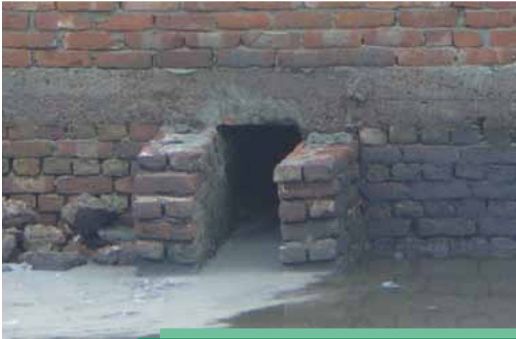
Tannery effluent flowing into surface waters
